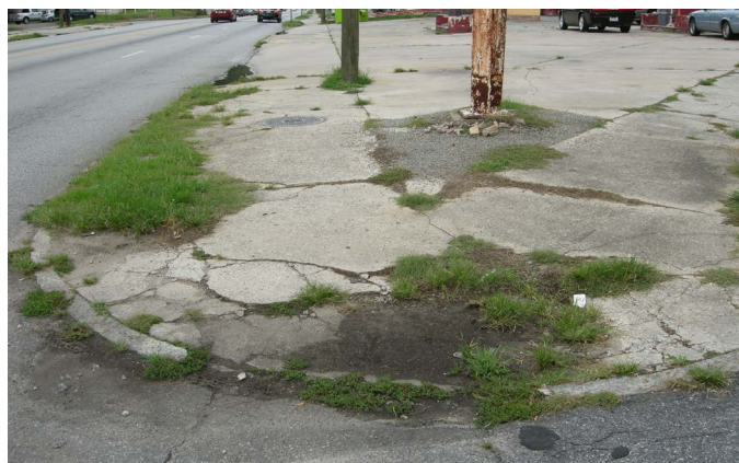
Deteriorating sidewalks are a safety hazard for pedestrians.
